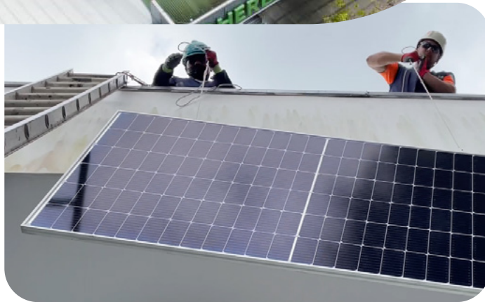
Costa Rica office solar array
